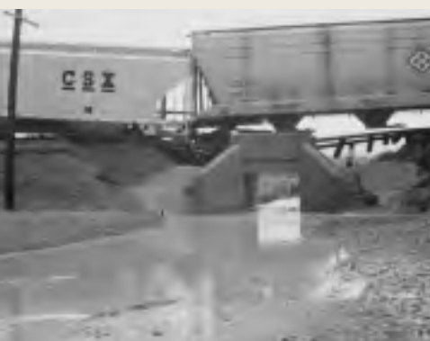
Erosion damage to rail line
