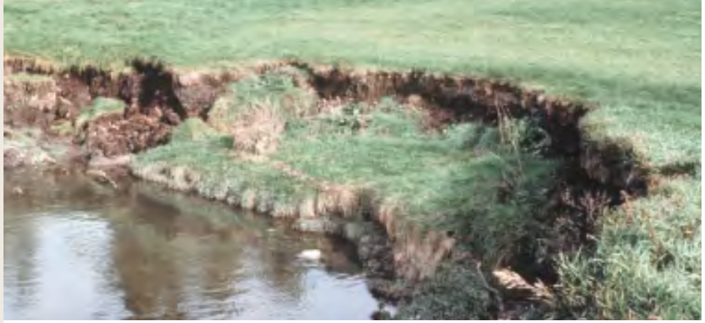
River bank erosion
